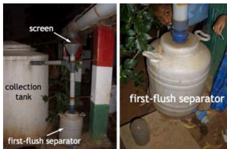
Figure 31. RTRWH at school in Misora, India. (Left: whole system with screen, first-flush separator and collection tank. Centre: screen. Right: first-flush separator.) Source: WAFLE (2010)
