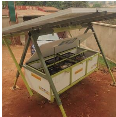
Figure 34: Sunblazer II Battery Charging Station, an example of the main structure (IEEE, 2017)
