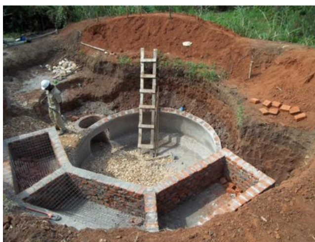
Figure 54: The Kasiisi School Biogas Digester (The Kasiisi Project, 2017)
