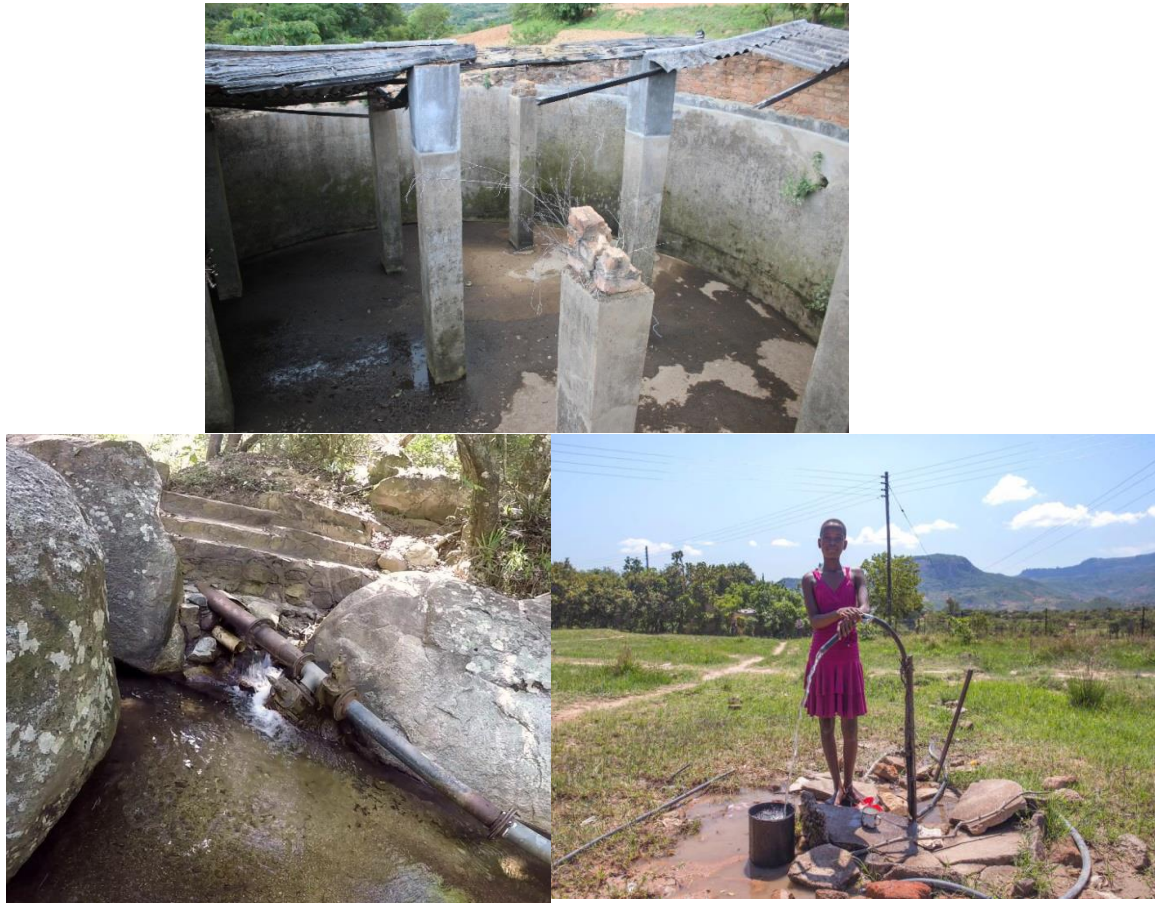
Figure 7: Main water tank in deteriorated conditions (top), water source in mountain (left), one main borehole (right) (photos by Leon Haupt and Sofia Gonçalves)
